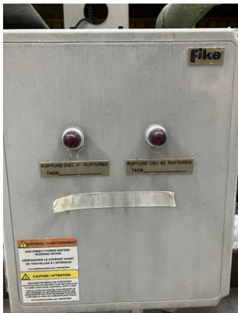
Figure 7. Decommissioned rupture discs.
