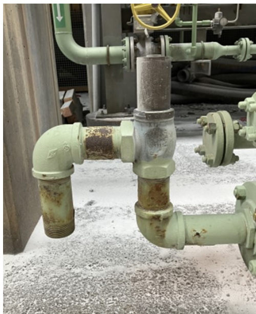
Figure 8. Process safety relief valve.
