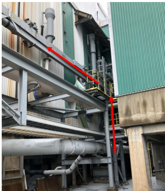
Figure 5. Outlet column feeding south HDPS.
