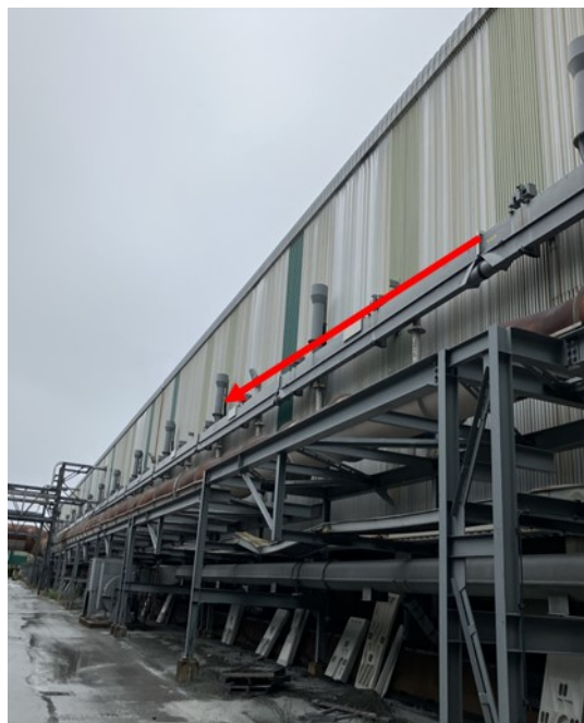
Figure 6. South HDPS branch
