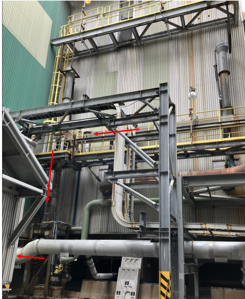
Figure 2. HDPS feeding the inlet side of the siphon.
